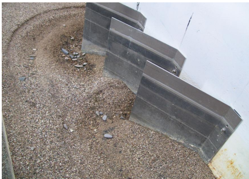
Figure 3. Picture of scoured bed surface
